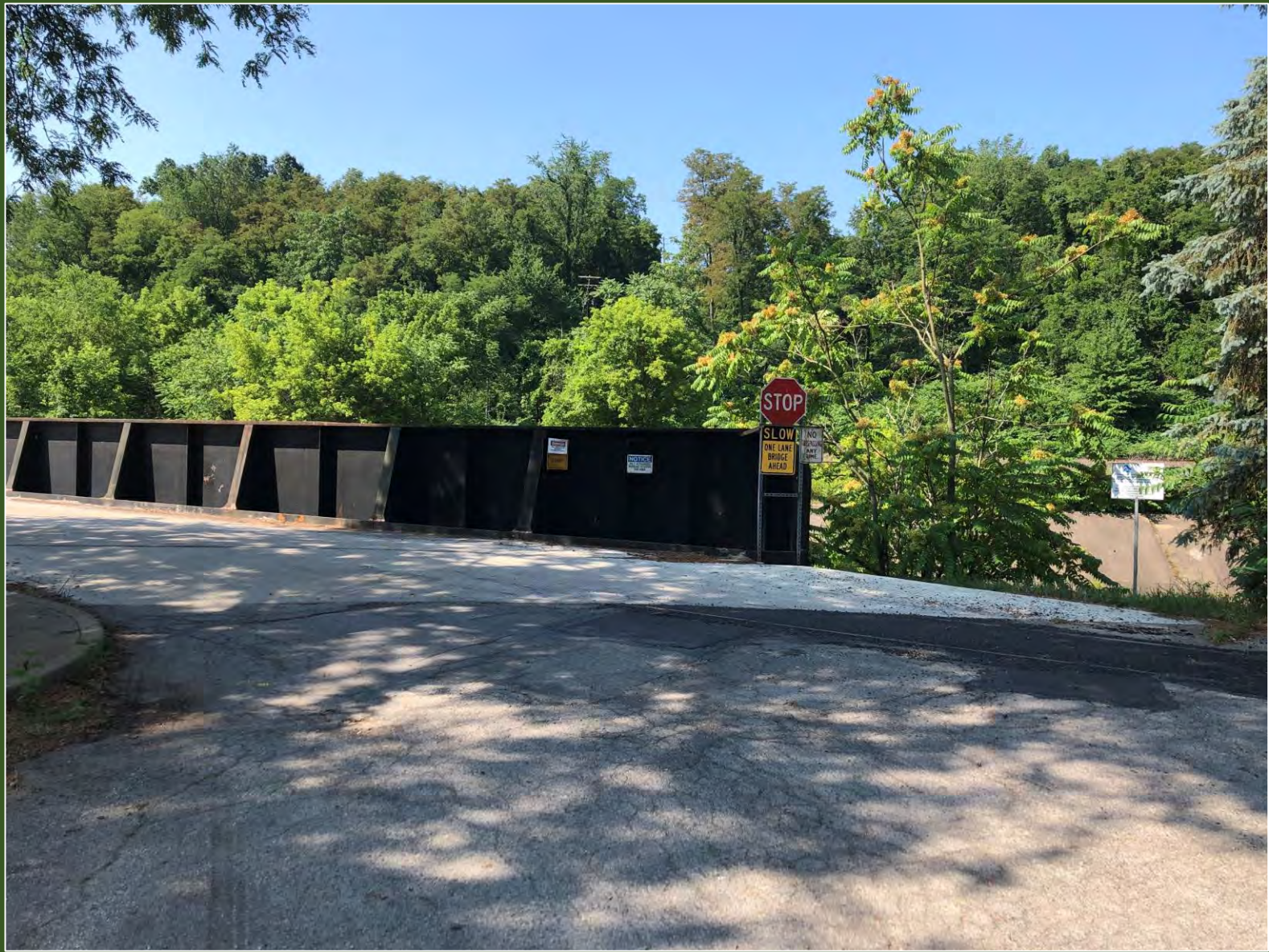
Airbrake Ave. & 4 th St. – Wilmerding View of Private Crossing over Turtle Creek Looking South
