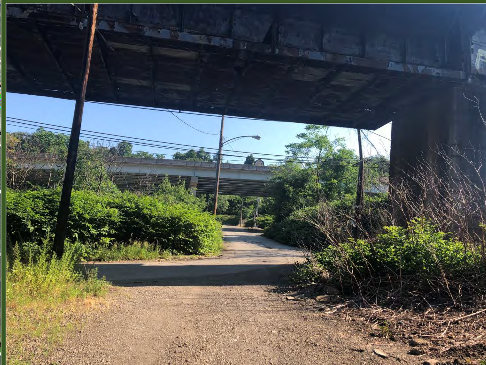
State Route 2183 & Main St. – East Pittsburgh View Looking North on Main St.
